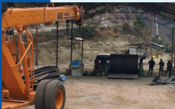
Hydromechanical workshop at Upper Naugarh
